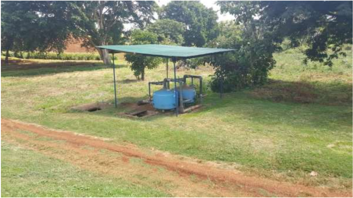
Water Filtration System
