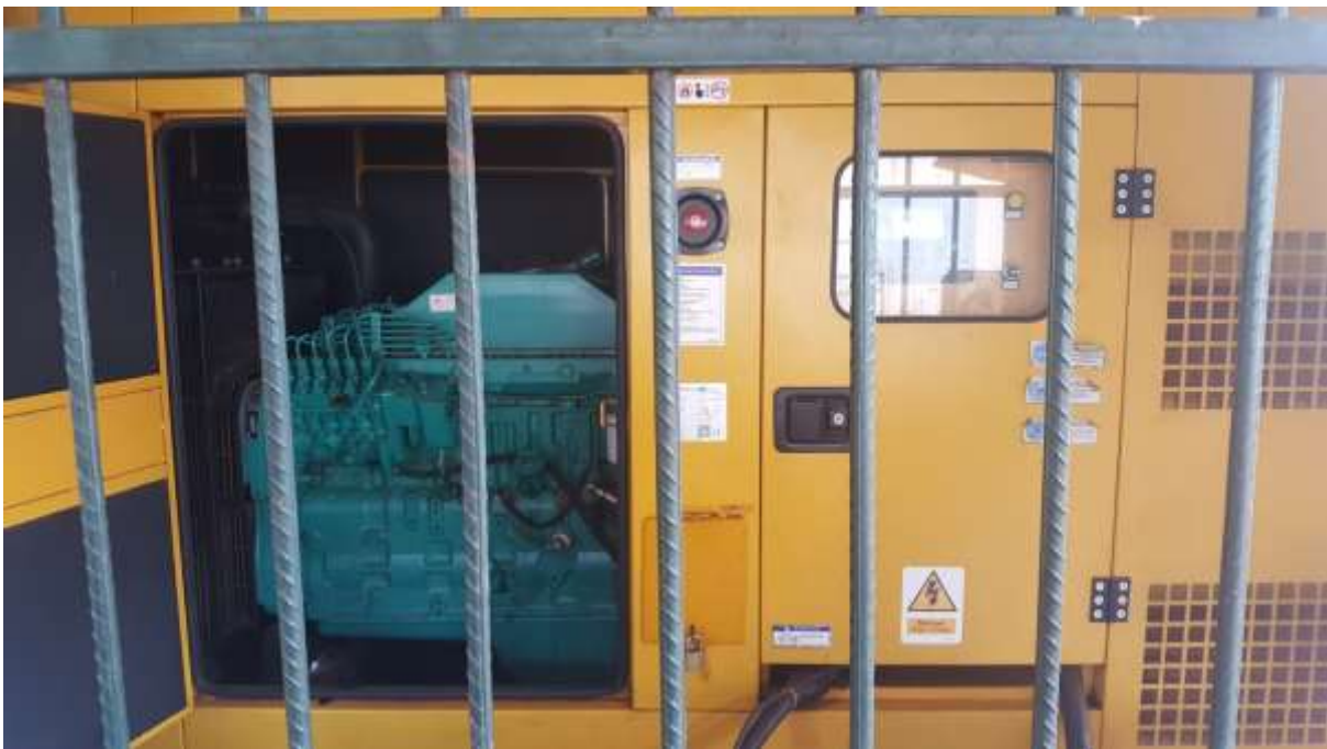
Generator 200kVa (Backup Power Supply)
