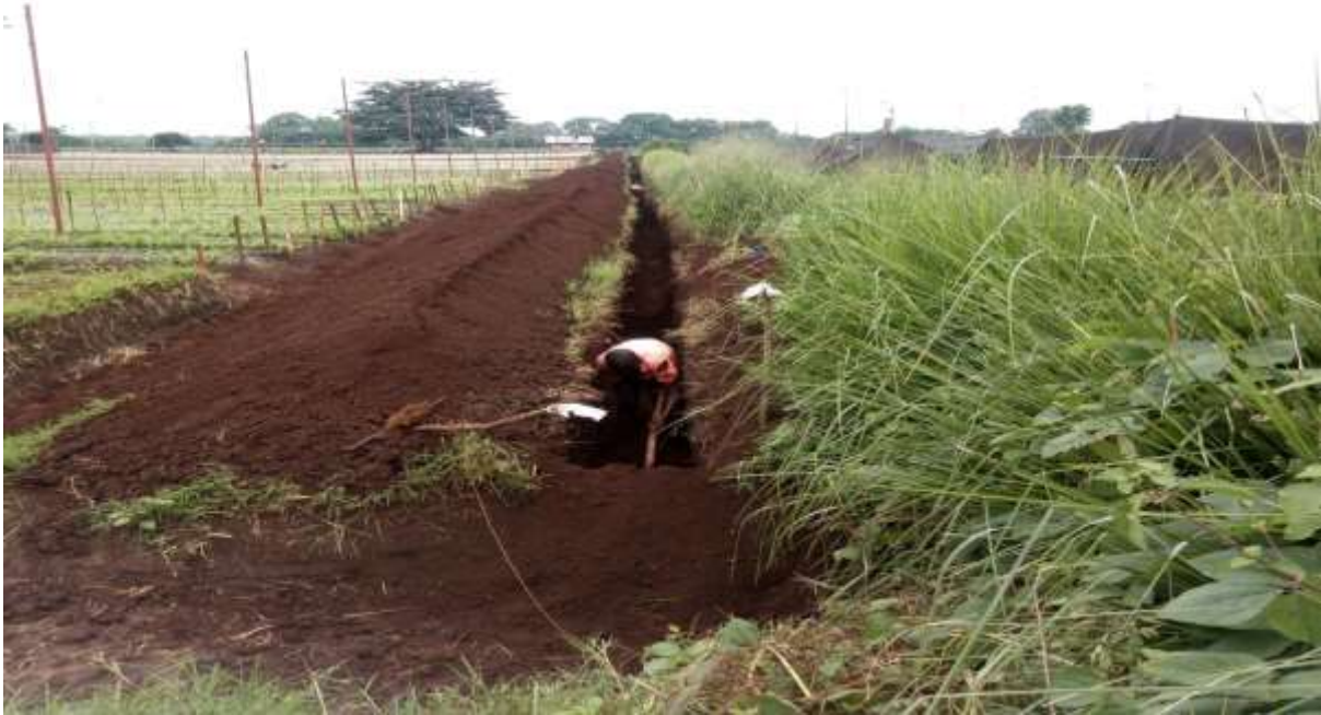
New Irrigation Mainline
