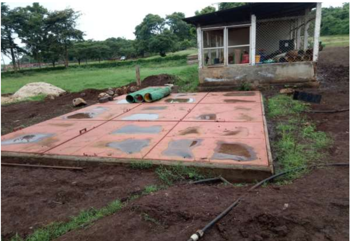
Chemical Deactivation Pit
