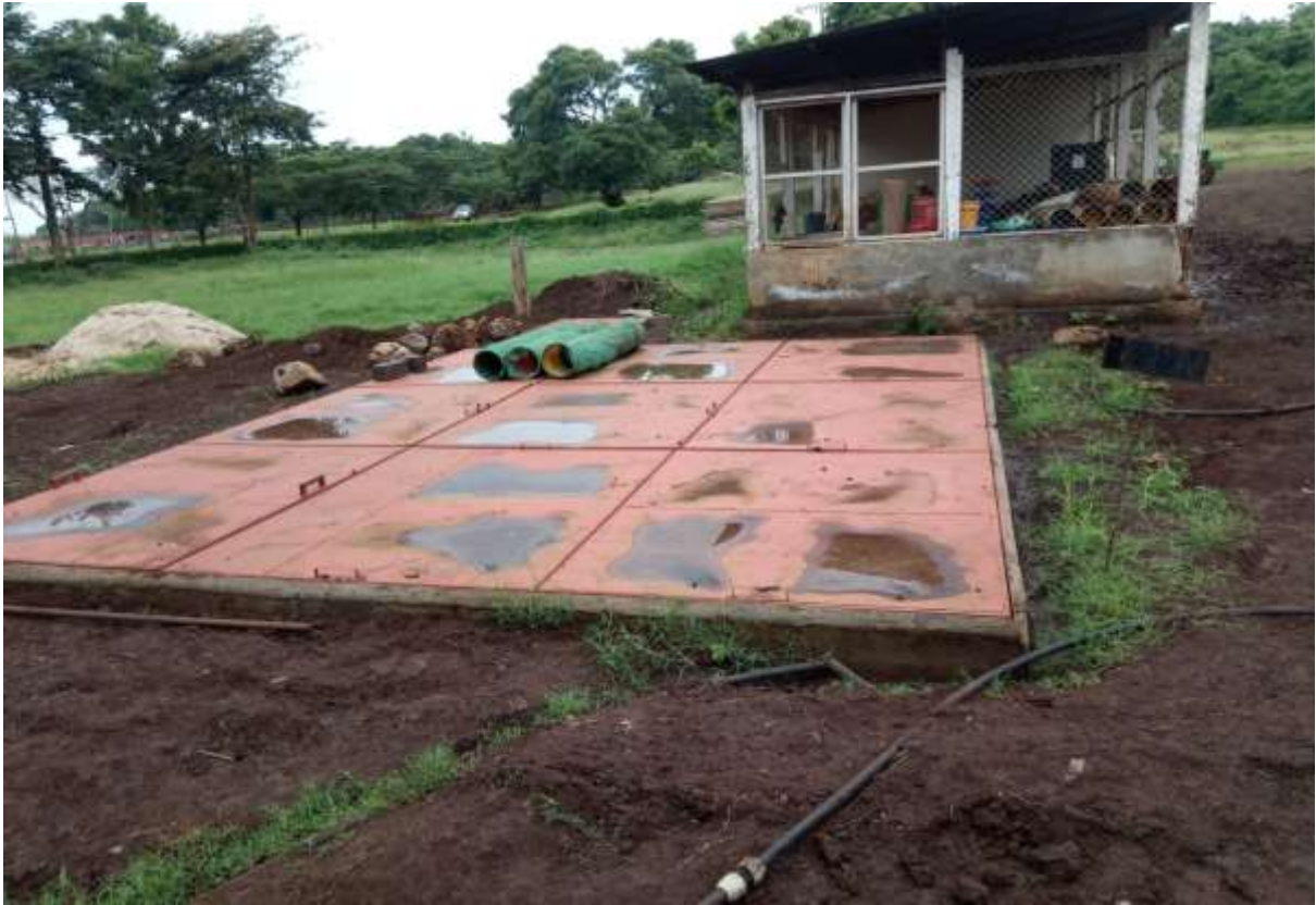
Chemical Deactivation Pit
