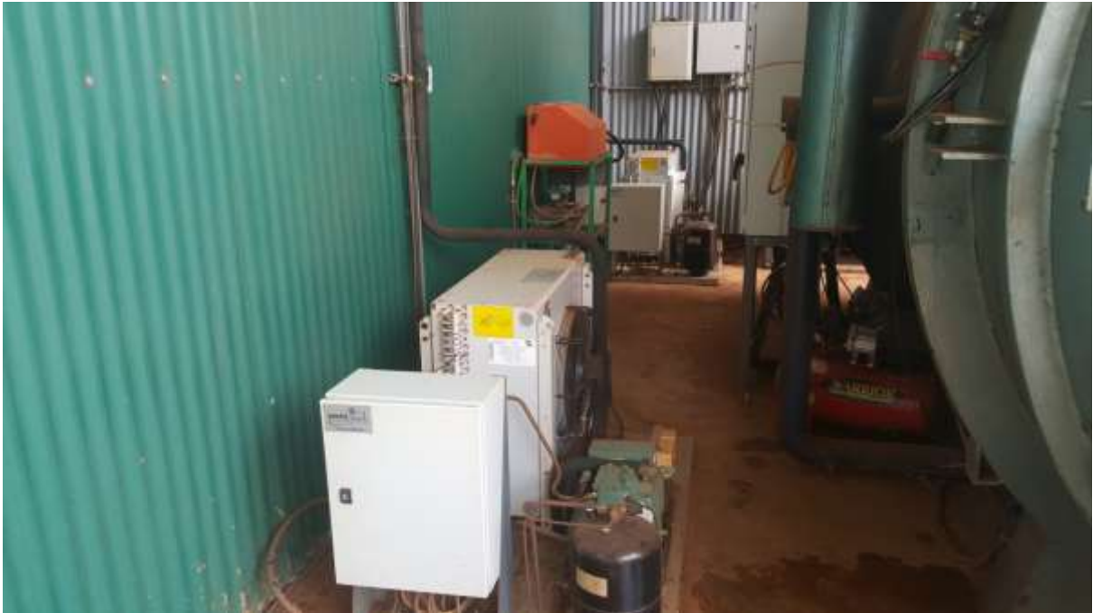
Coldroom Equipment & Misting System
