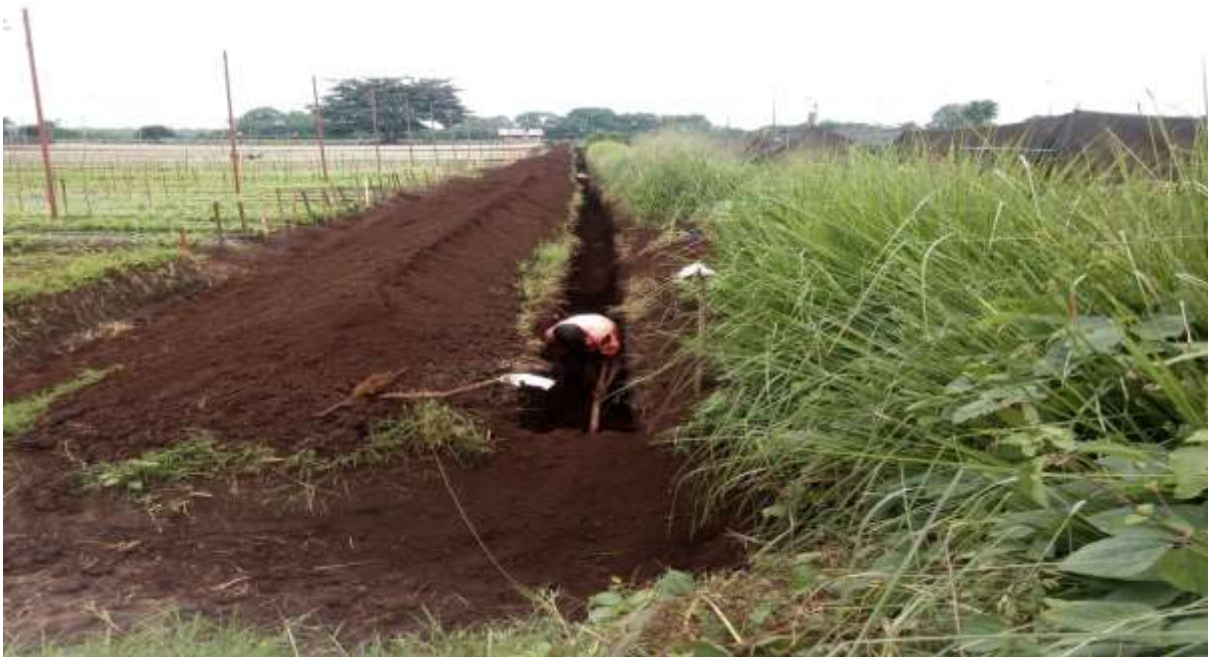
New Irrigation Mainline
