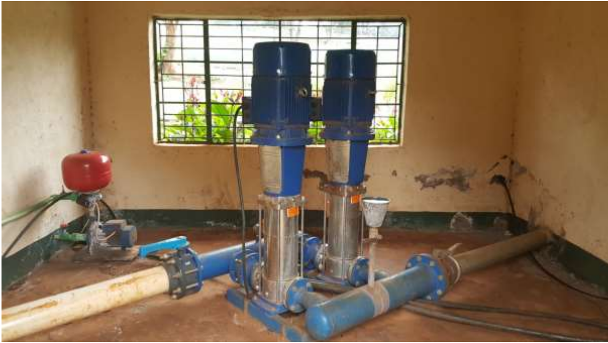
Pump House Interior.
