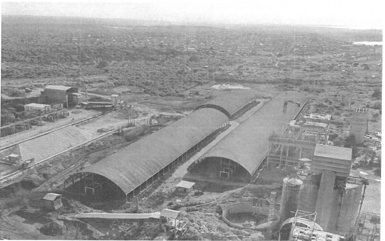
Aerial picture of the on-going construction of the cement grinding factory at Maweni
