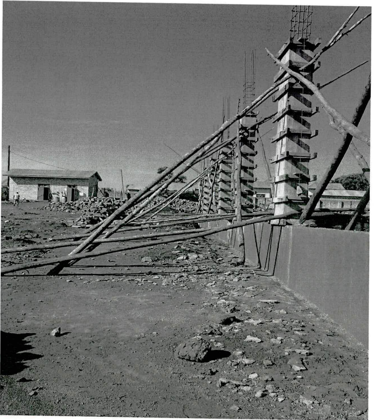
View of part of factory building of GDM Company Limited under construction
