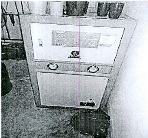
Water Chiller Machine
