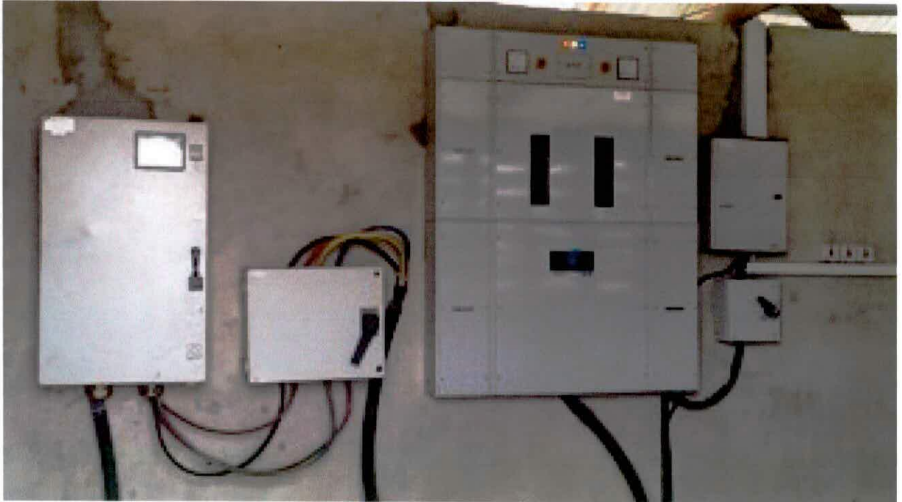
POWER DISTRIBUTION PANEL
