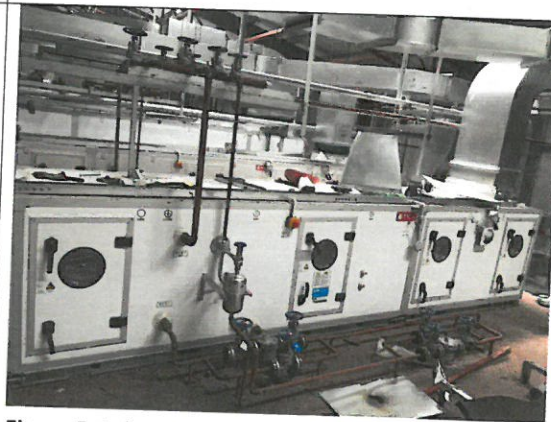
Figure 5: Laboratory AHU at site
