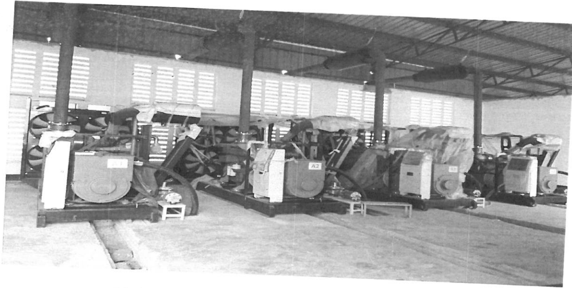
Plate 2: Gas generators installed in the facility
