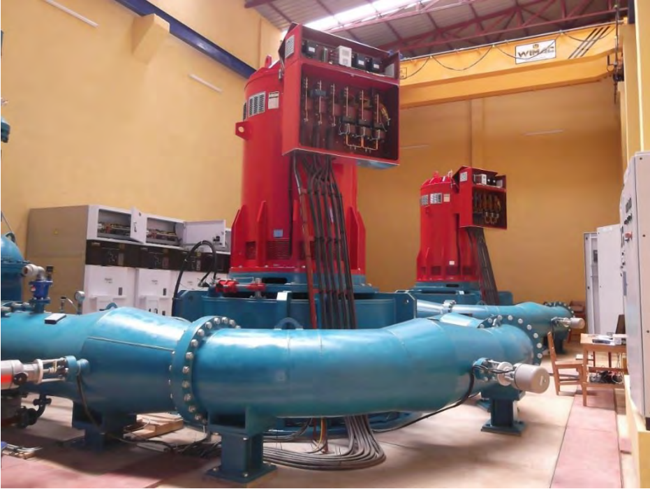
Figure 36. Example of two vertical Pelton turbines with 5 nozzles
