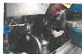
The technicians also inspect the hydraulic systems including the oil filter of the gearbox.
