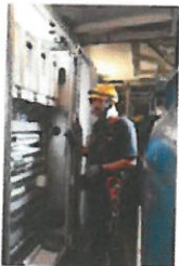
The technician takes a look at the switch cabinet in the nacelle.
