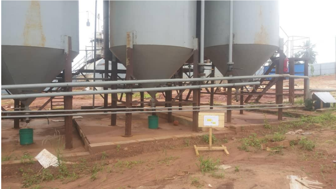
Sign Board @ Oil Purification Tanks' Side. (Unauthorized Person Prohibited)
