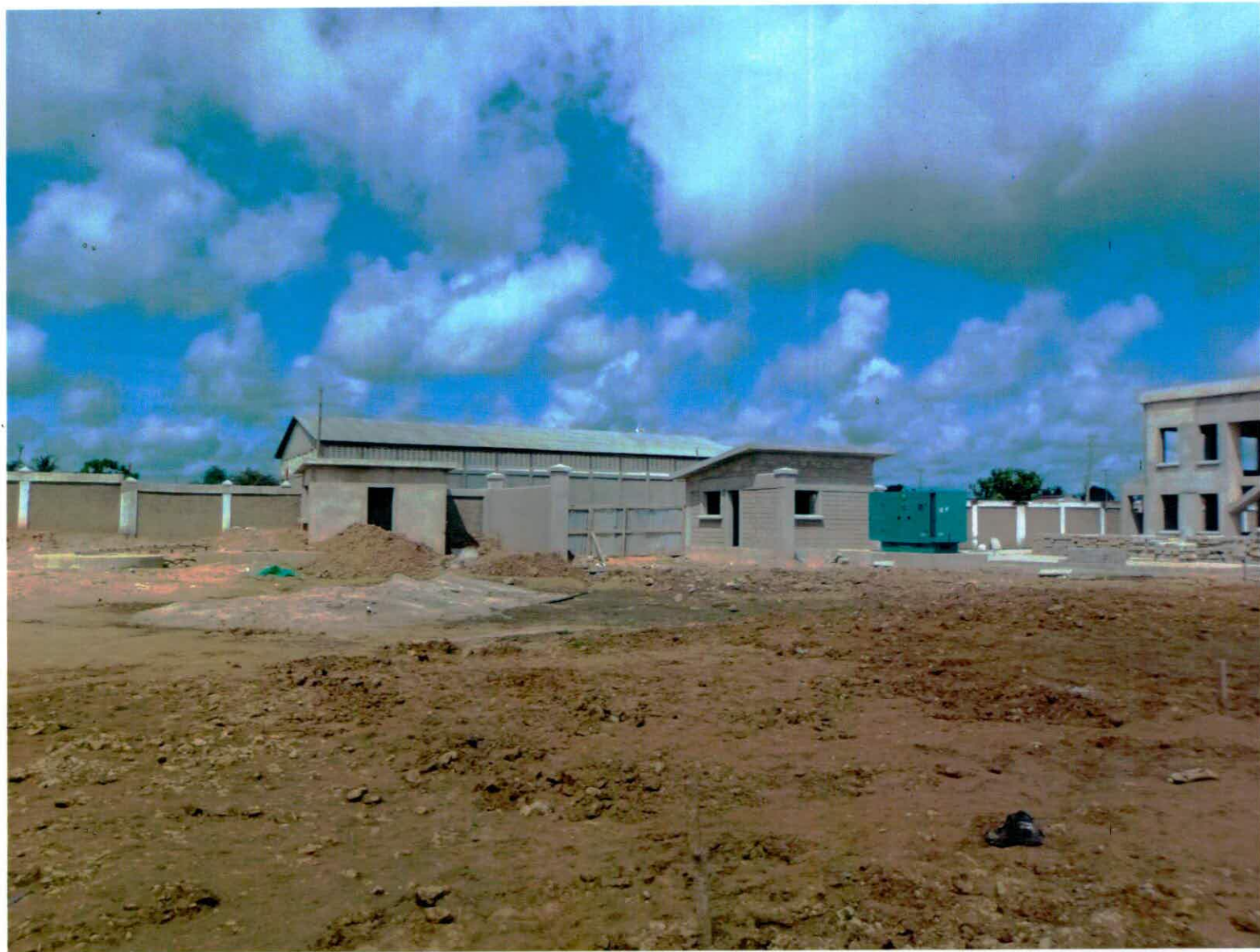
Electric room, generator , guest room and gates
