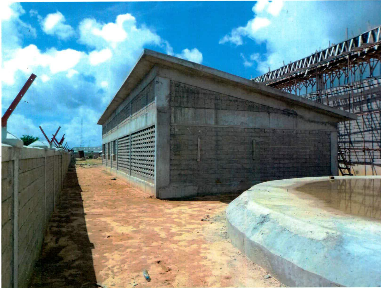
Firefighting room from back side veiw
