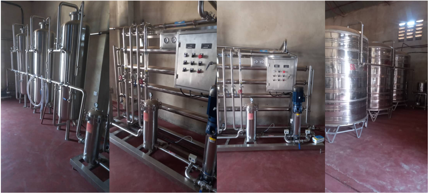
Reverse Osmosis water treatment plant for production 10,000 Ltrs per hour of purified water and also stainless steel temporary product storage tanks.
