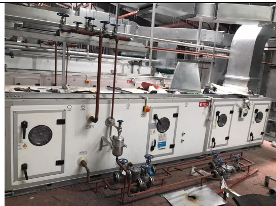
Figure 5: Laboratory AHU at site
