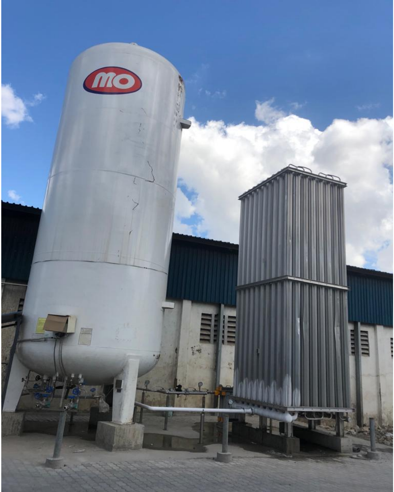
2. Carbon dioxide tank
