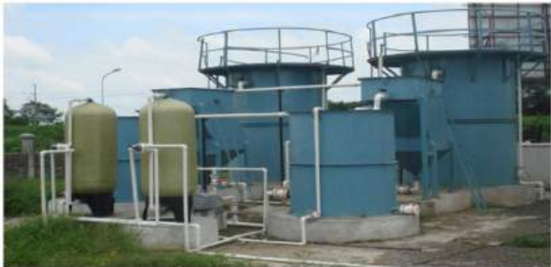
Effluent Treatment Plant
