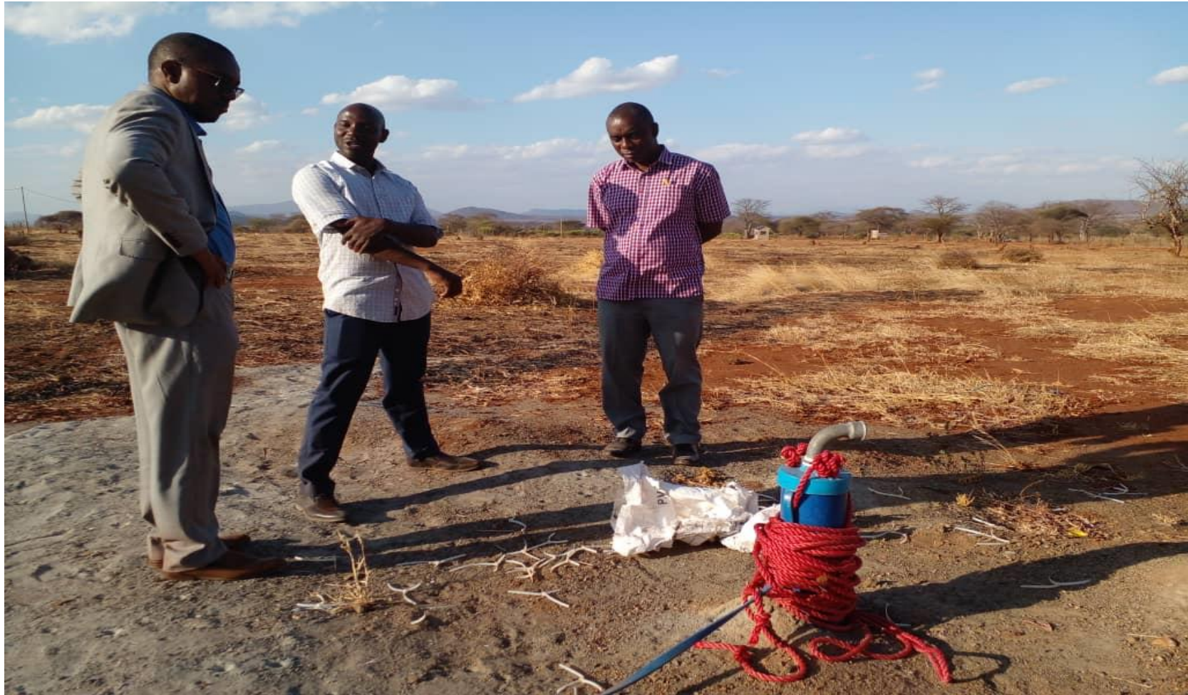
Discussion at the bore hole drilled for supply of water for the project, the drilled well is expected to have a capacity of about 10,000 litres of water per hour.
