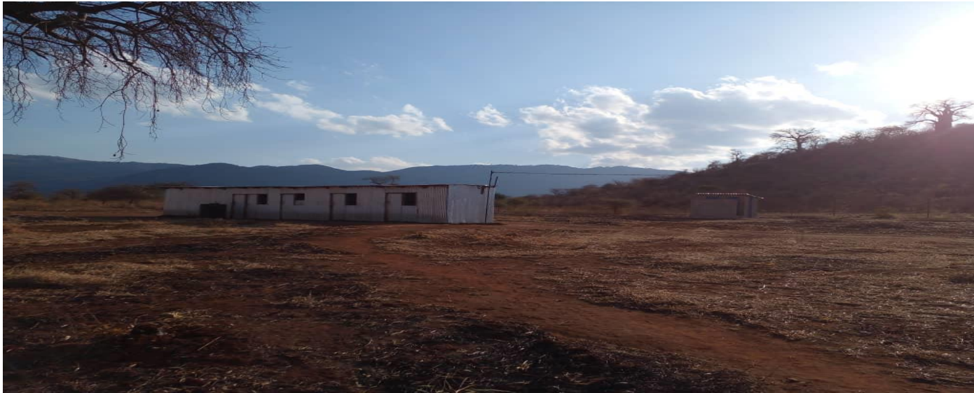
Constructed temporary house for materials, wokers' office and security guards(above), Weight Bridge cabin(below)
