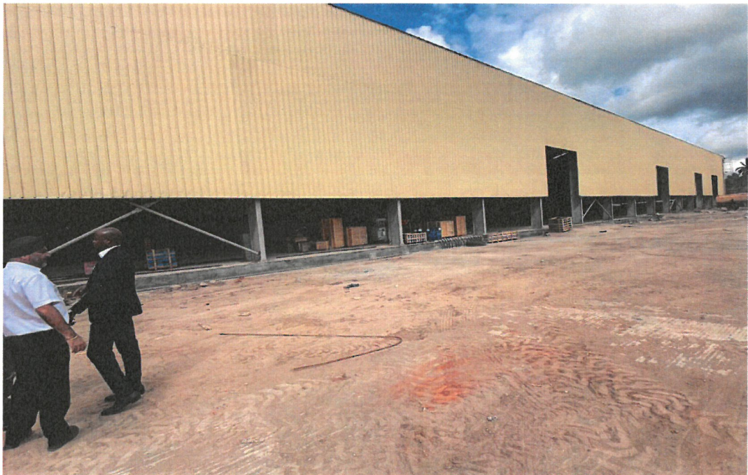
Extension of the of the new warehouse/shade for storage of scrapers and cutting of scrapers as per NEMC requirements
