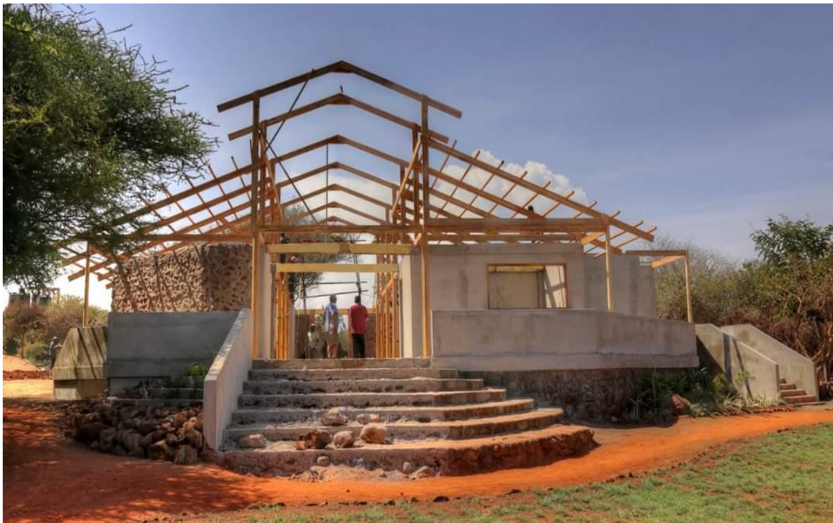
Figure 7: Construction of the Main Building of Manyara Safari Lodge is already underway, thanks to Lodge Creations.
