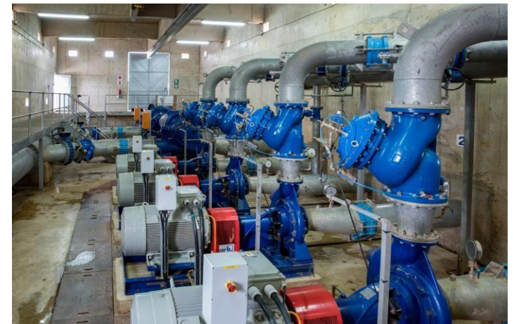
One of KSL's pump stations
