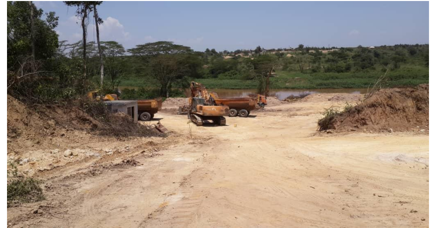
Preparation of the area where the bridge will be assembled and installed.
