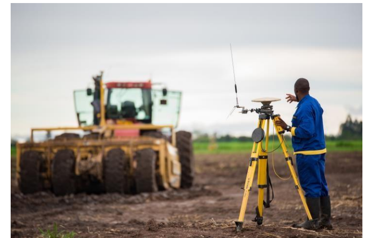
Step 5/6: GPS controlled machine tractors and scrapers levelling the land, followed by ripping operation
