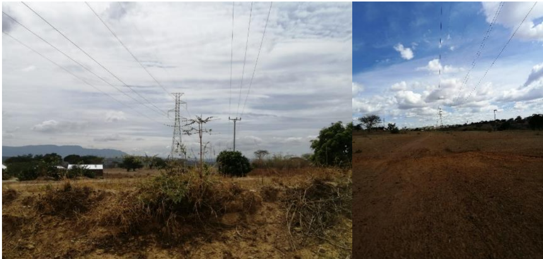
Figure 11: Existing 220-kV and 33-kV lines (Source AFA)
