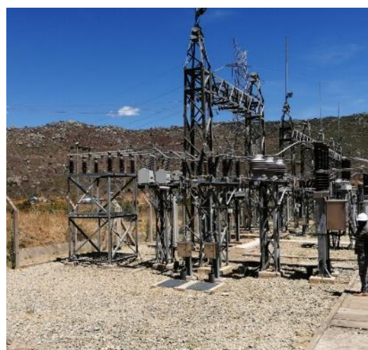
Substation 33-kV Bays
