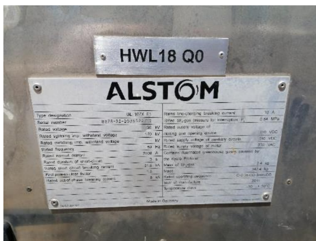
Circuit Breaker Plate of Spare Feeder
