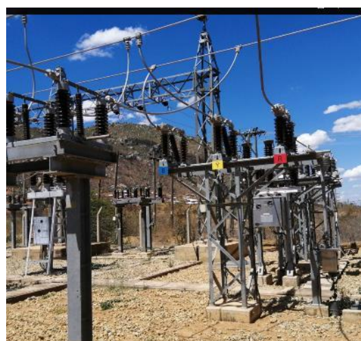
33-kV Spare Feeder
