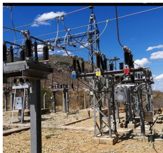
33-kV Spare Feeder
