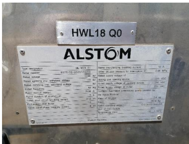
Circuit Breaker Plate of Spare Feeder
