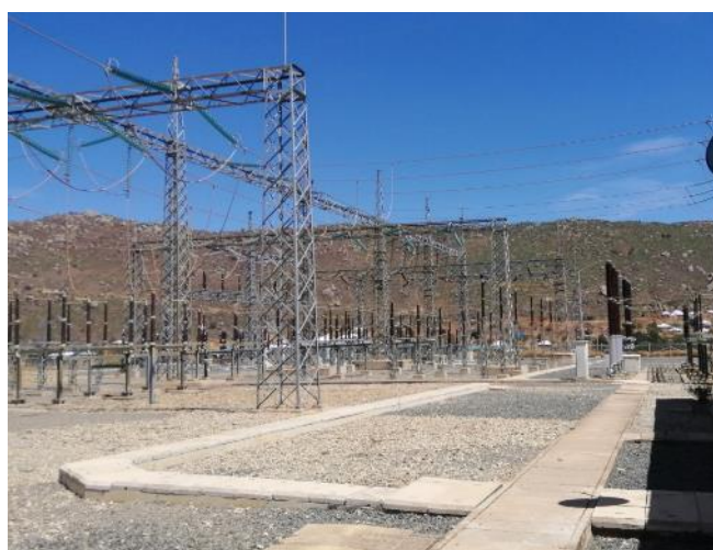
Substation 220-kV Bays
