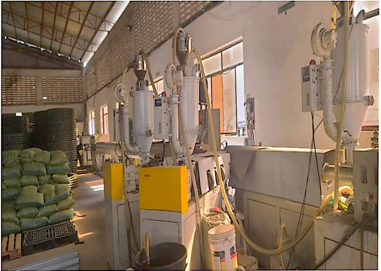
Coil Pipe Machine
