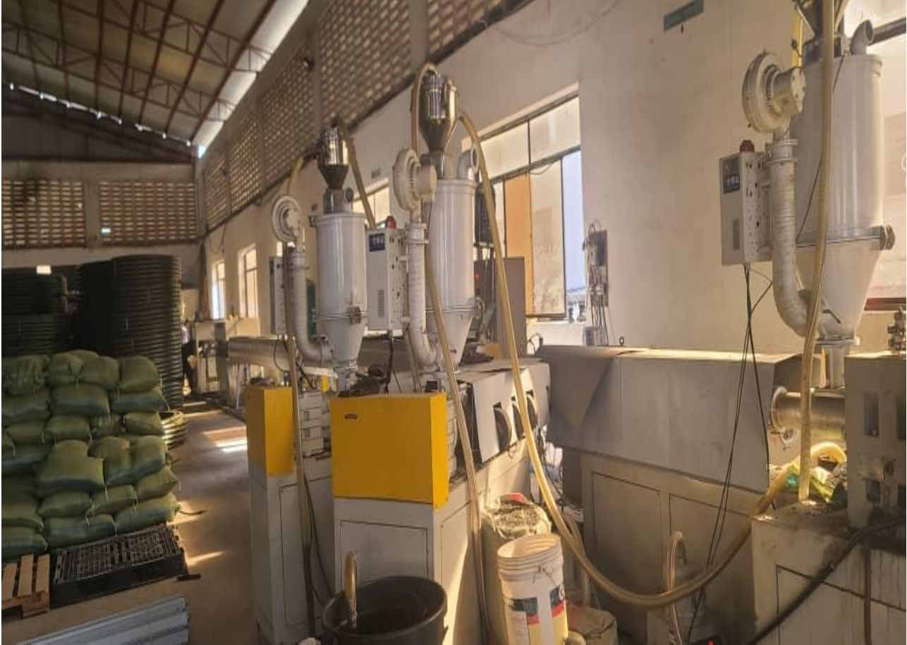
Coil Pipe Machine
