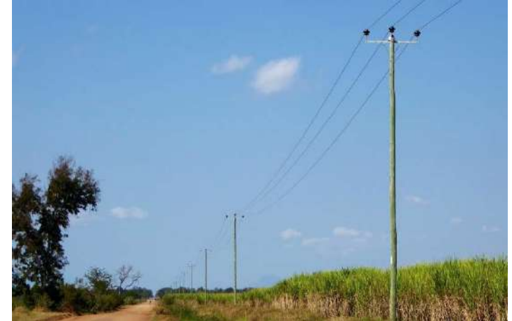
Part of the power infrastructure installed by MSE.
