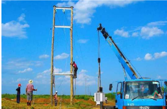
MSE has installed power infrastructure at the estate.
