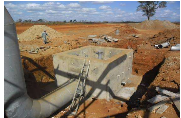
Water pipes as part of the irrigation infrastructure
