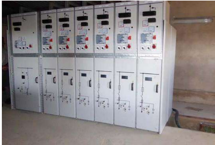
Power equipment at MSE
