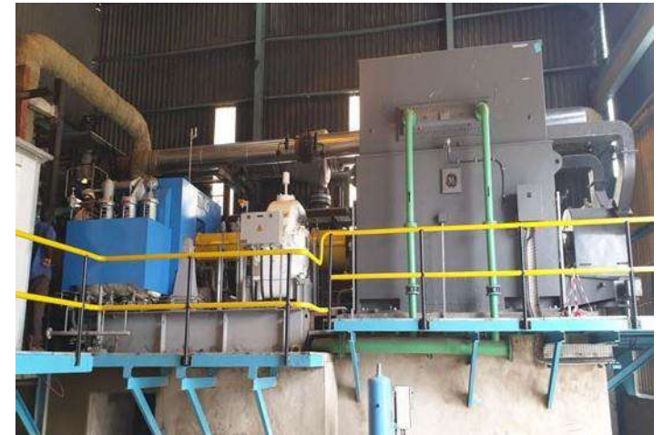
New 15 MW TA generating set at MSE.
