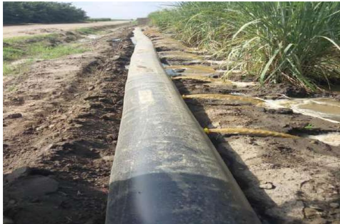
New lay flat irrigation system at work.
