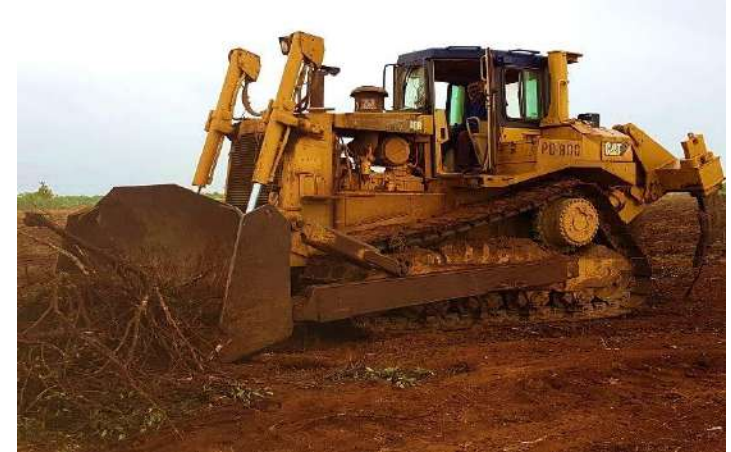
Step 2/3: A second clearing process to knock down the anthills, Ripping and initial levelling of the land
