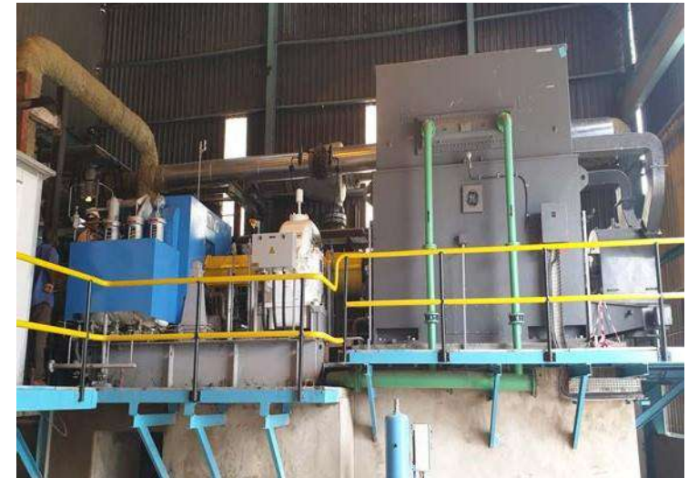
New 15 MW TA generating set at MSE.
