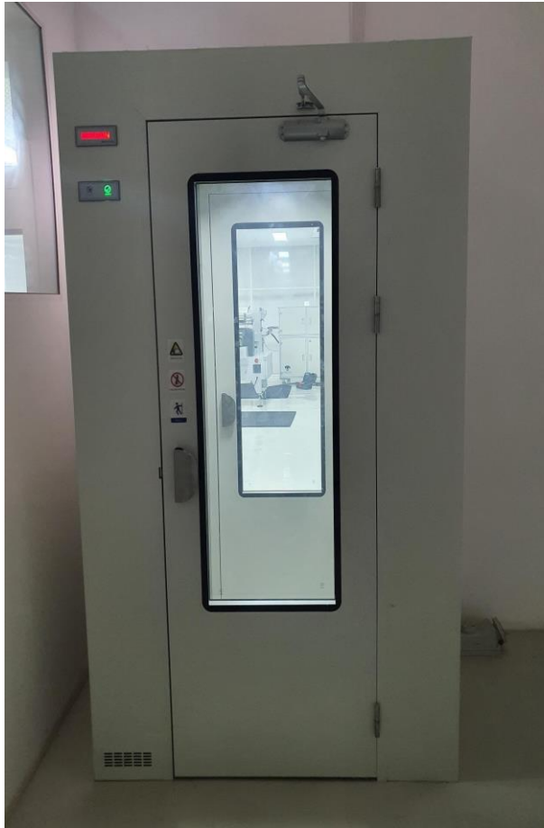
Figure 2: Photo of cleanroom air shower entrance
