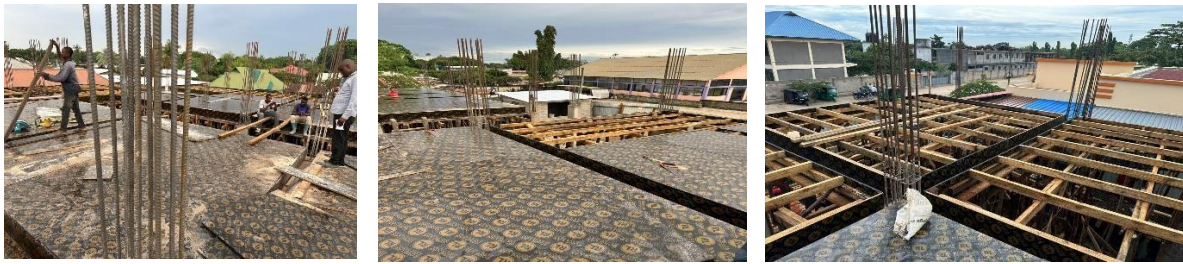
Current overview status of the Medical Facility main building on-going construction works
