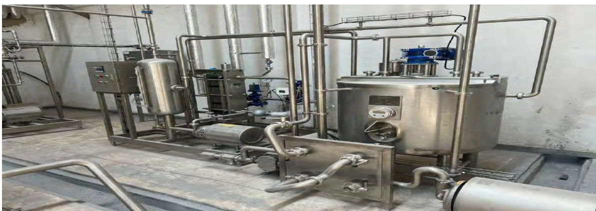
Figure 2: 20,000 LTRS Milk Processing Plant Installed at Karagwe, Kihanga Industrial Park (Inside View)
