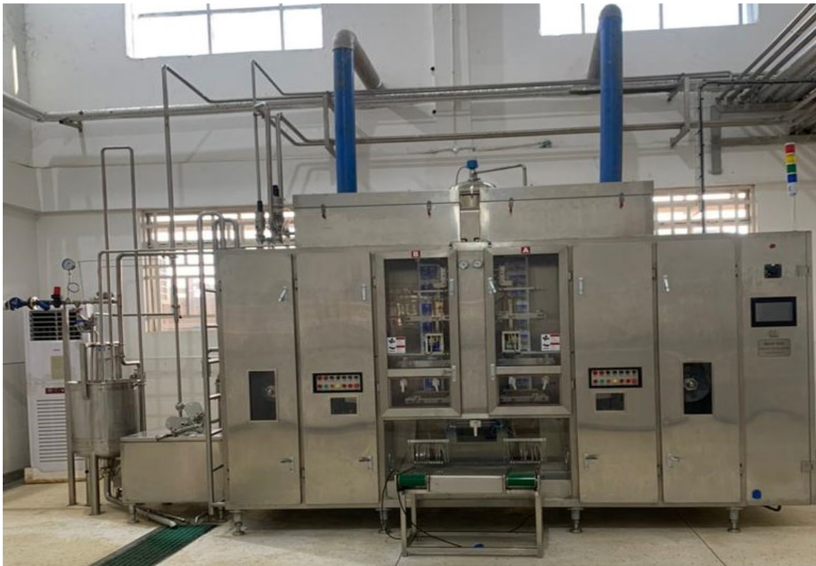
Figure 4: Acquired & Installed UHT Milk Processing Plant
