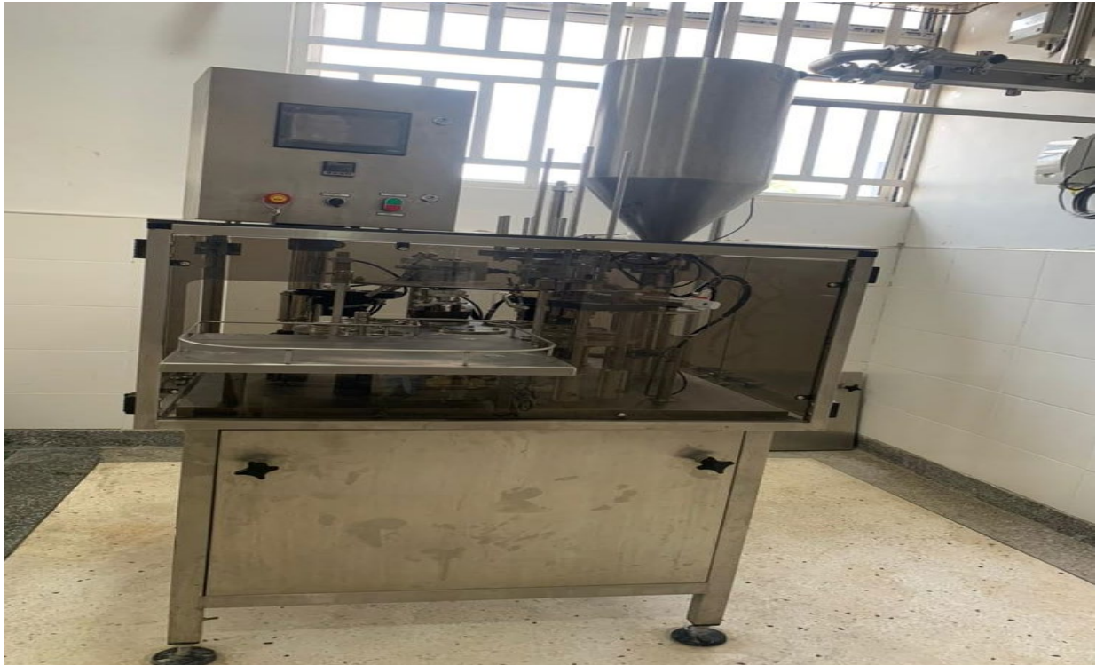
Figure 5: Installed Yoghurt Packing Unit
