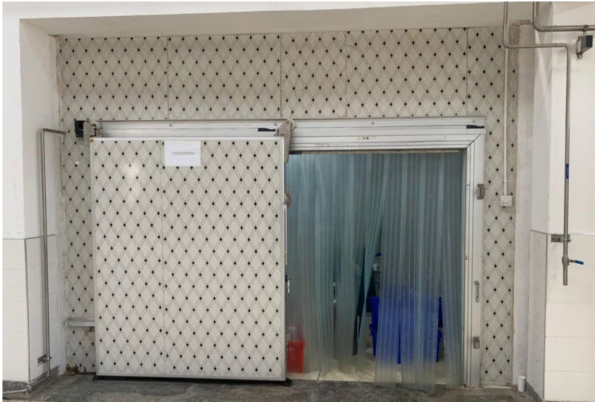
Figure 7: Installed Cold-room for cooling Milk processed products
