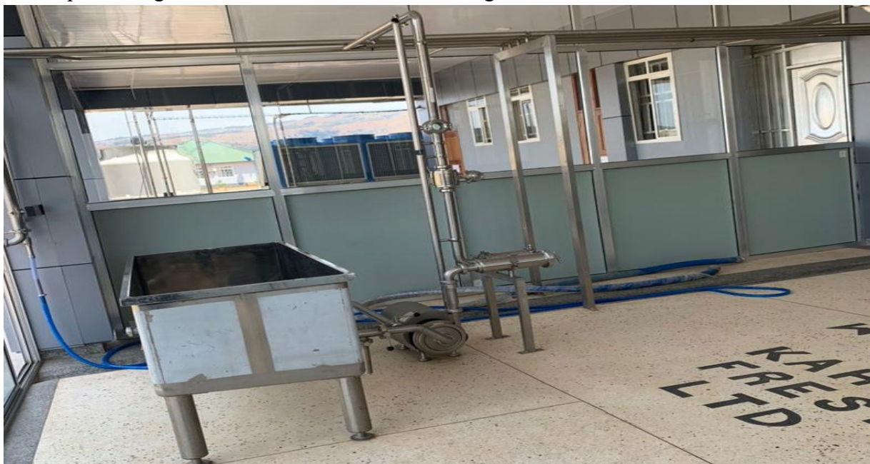
Figure 8: Raw Milk Receiving Point at the factory (Front section)
