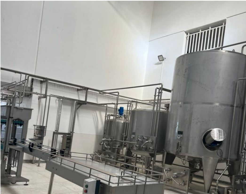
MILK PROCESSING PLANT PROJECT: INSIDE VIEW- MILK PROCESSING UNIT UNIT
