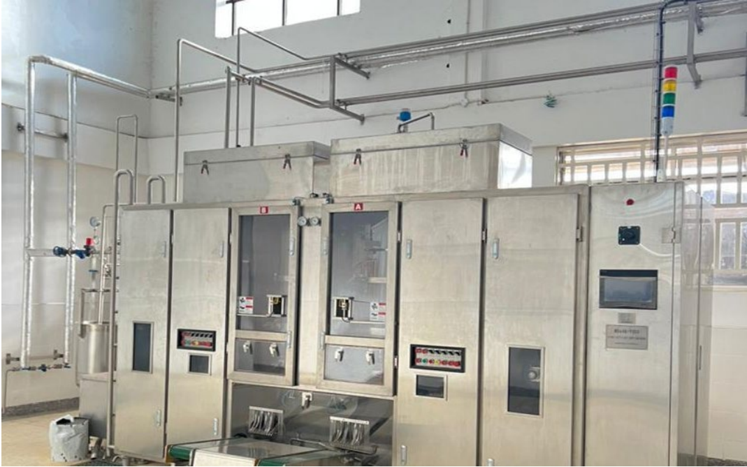
MILK PROCESSING PLANT PROJECT: INSIDE VIEW- UHT UNIT
