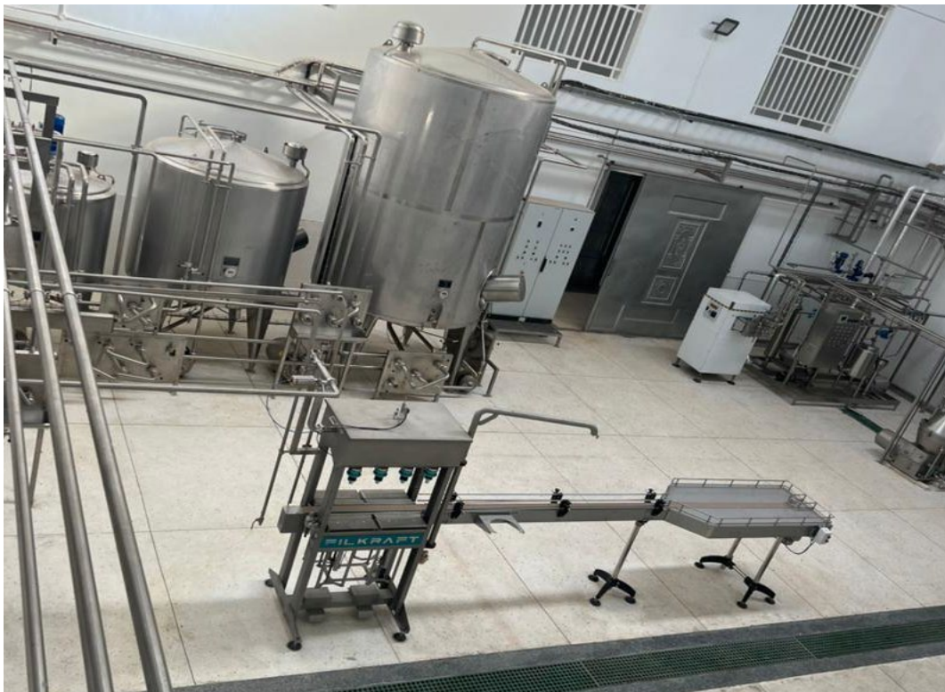
MILK PROCESSING PLANT PROJECT: INSIDE YOGHURT PROCESSING SECTION
