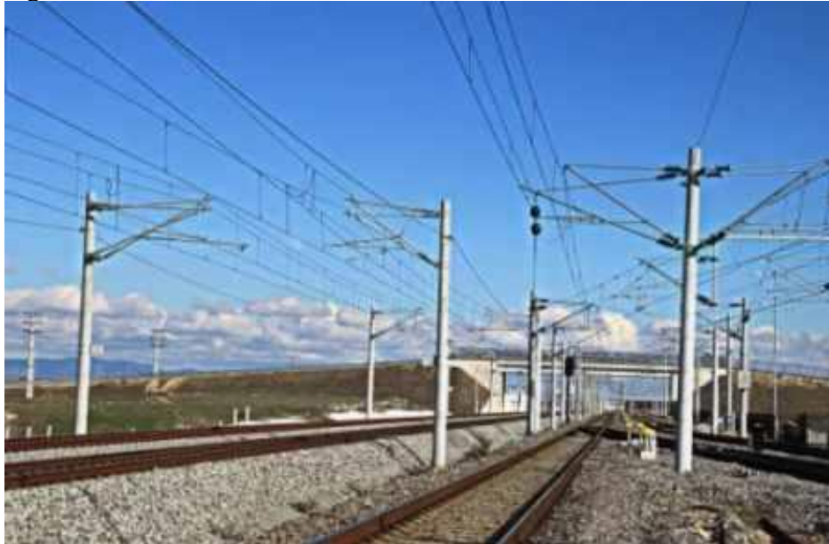
Figure 5: Picture of Concrete Poles in Use for Transmission of Electric Lines
