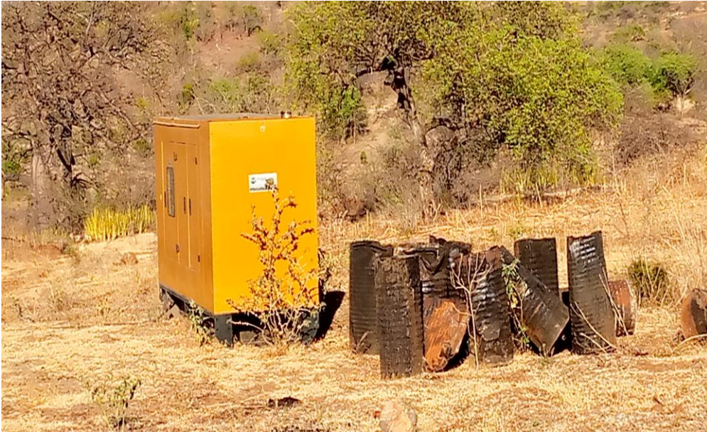
Installed Generator for backup electricity during the shortage of TANESCO power
