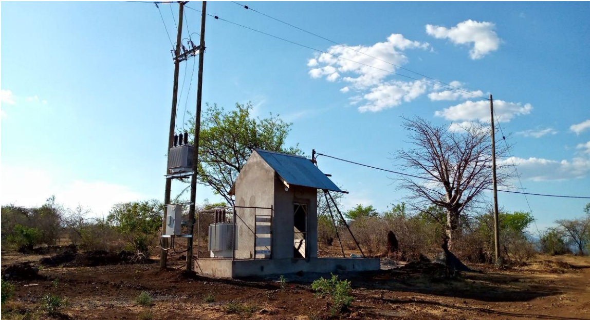
Installed Company generator and TANESCO electricity
