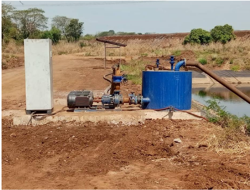
Photo 15: Return water pump located at TSF area
