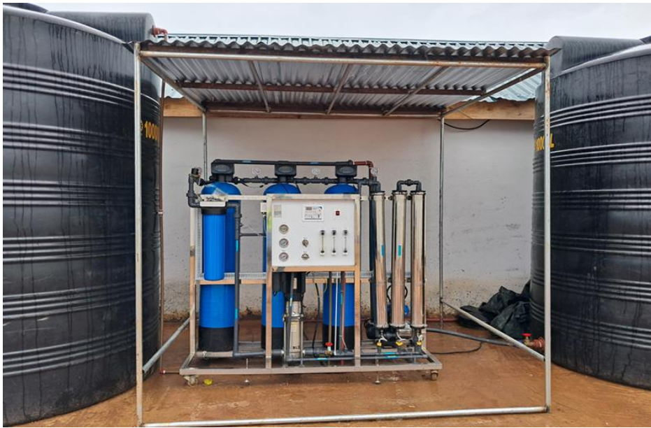
Photo 5: Reverse Osmosis Water Treatment Plant at Lindi Jumbo Mine Site
