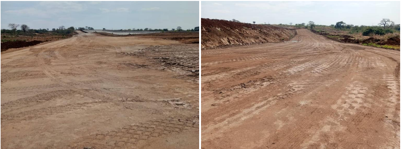
Photo 13: Lift one embankments around the TSF area out at Lindi Jumbo Mine Site
