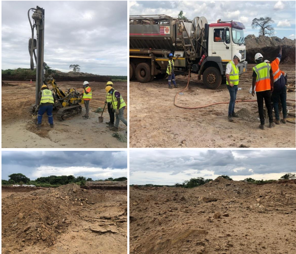
Photo 12: Open Pit drilling and blasting activities were carried out at Lindi Jumbo Mine Site
