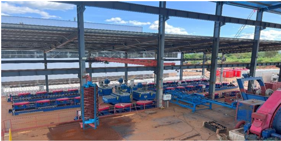
Photo 8: Flotation section commissioning at Lindi Jumbo Mine Site
