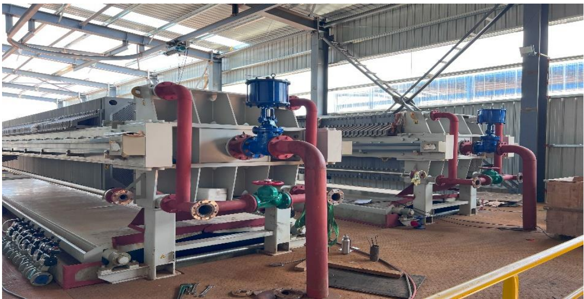
Photo 9: Filtration section commissioning at Lindi Jumbo Mine Site
