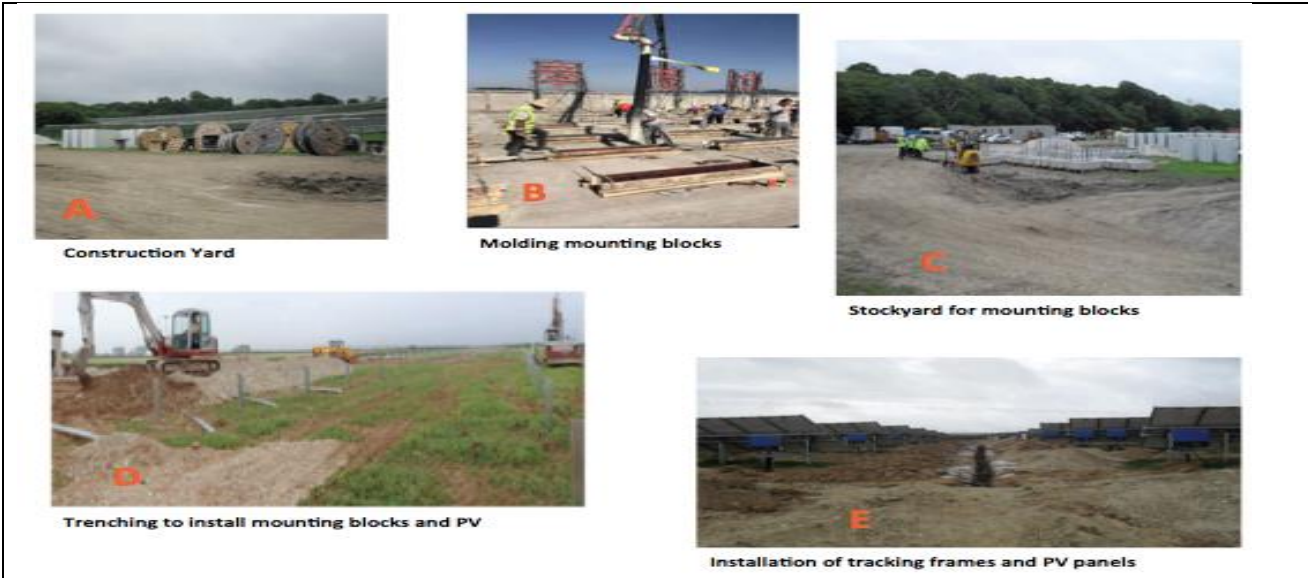
Figure 9: Project Site and PV mounting, molding and Installation A Construction Camp yard B Molding cement blocks for the PV Solar frame installations C Stockyard for mounting blocks before installation into field D Trenching to instal mounting blocks for PV Frames E Installation of tracking frames and Mono Solar Panels
