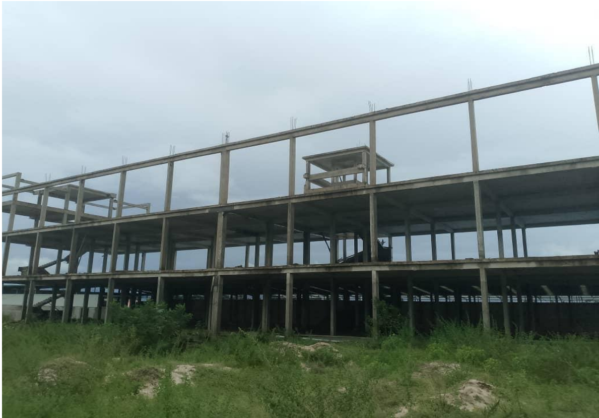
Photos showing front view of the framed structure of an office building.
