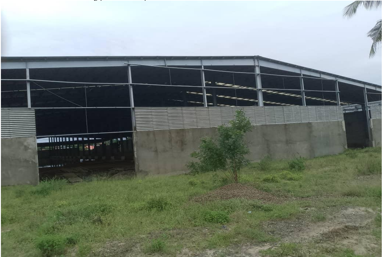
Photo showing the warehouse building awaiting finishings and decorations such as the glass work, painting etc Kigamboni Project
