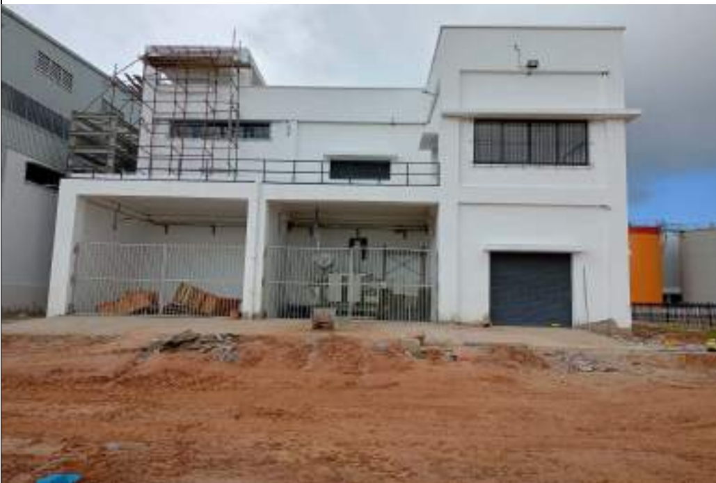
Figure 3-Sub station over all view
