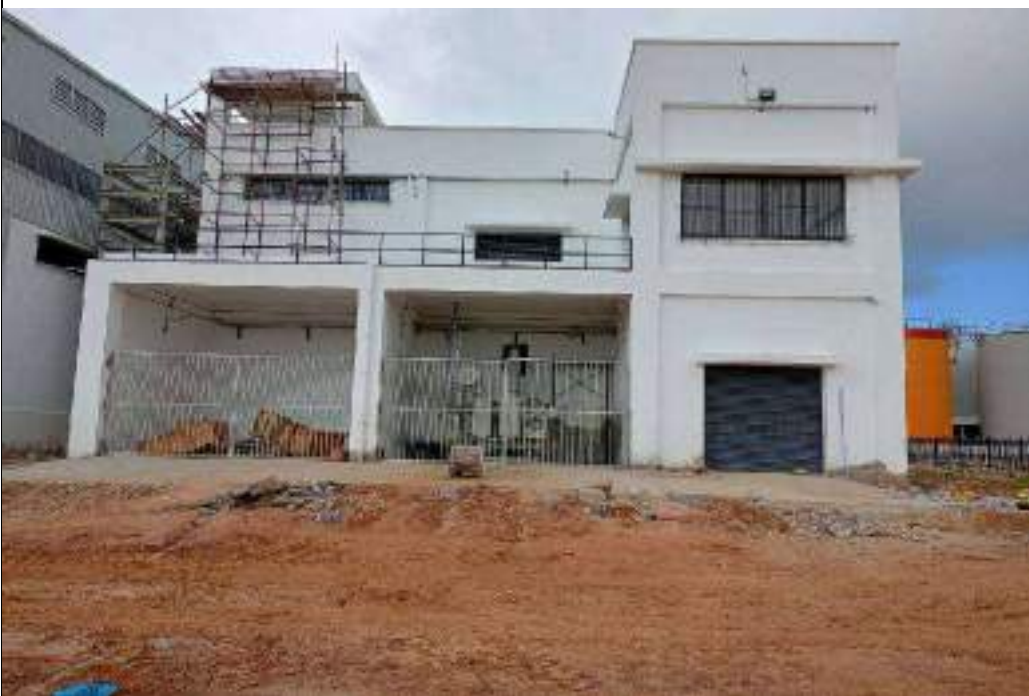
Figure 3-Sub station over all view
