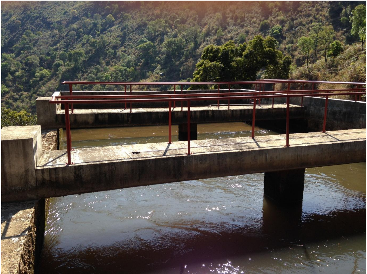
Picture 2: Sediment tank
