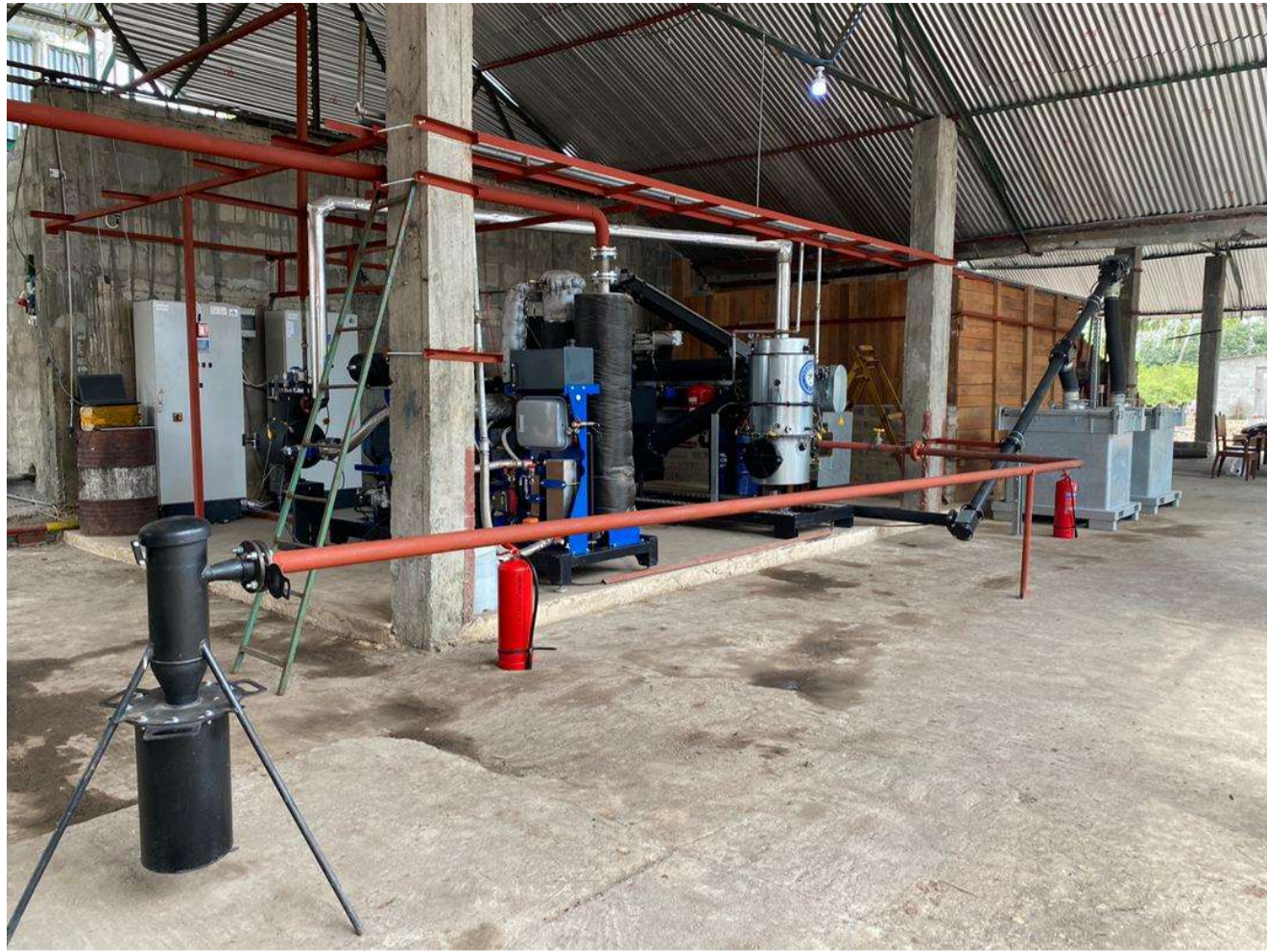
50 KW plant on Mafia Island Commissioned in July 2021.
