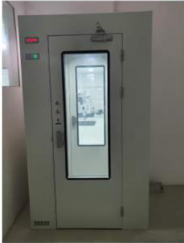
Figure 2: Photo of cleanroom air shower entrance
