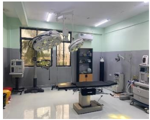
Major Theater equipment
