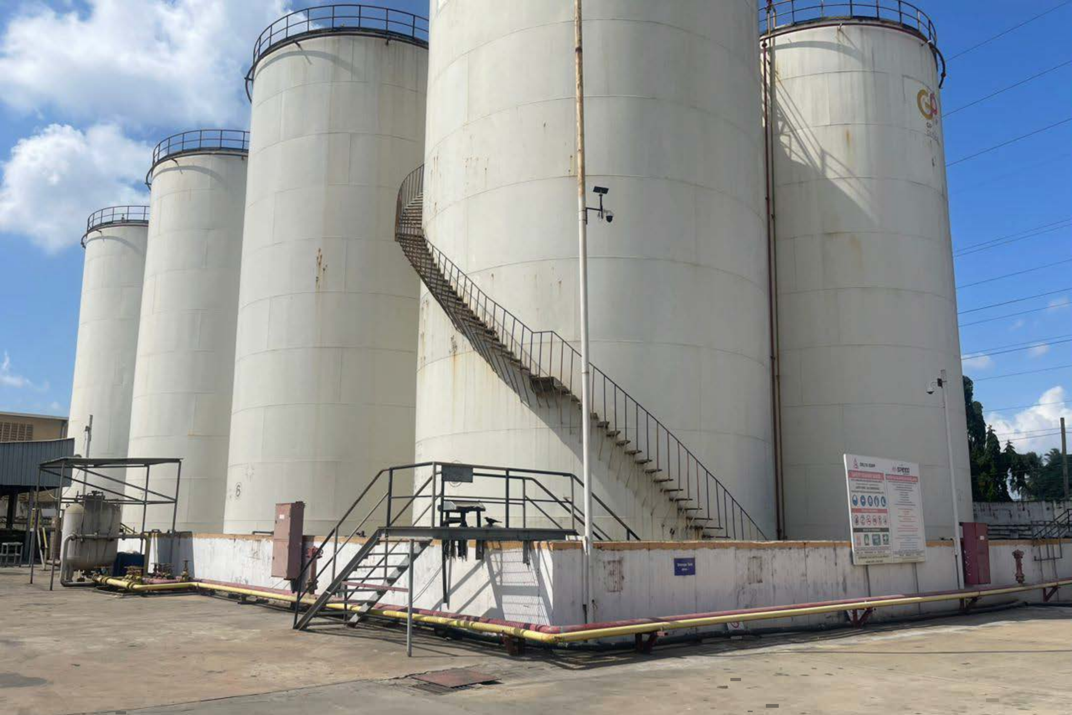
STORAGE TANKS ALL VIEW
