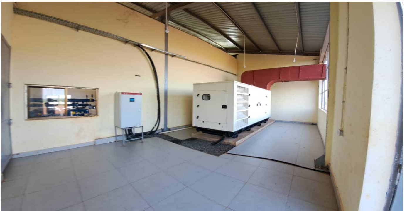
Back up generator -300 KVa as power source in Intake-1
