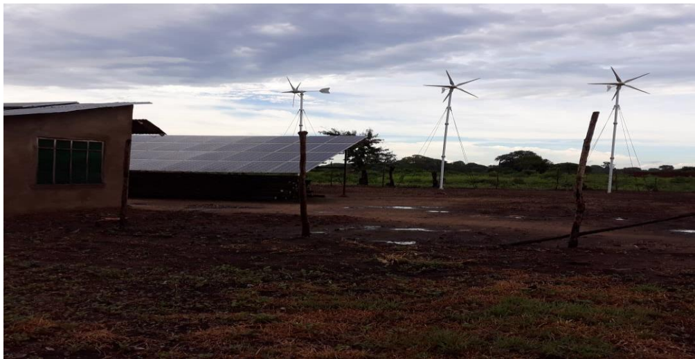
Figure 1: Nanjirinji hybrid (solar and wind) miniGrid deployed using LRTC2014 funding
