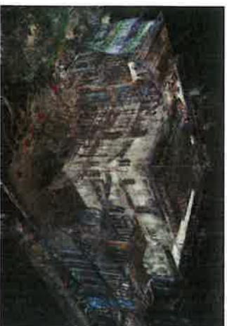
3D Photographs (re) of partially collapsed building by Zanzibar Cape Town
