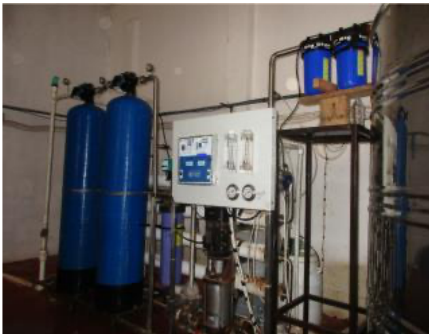
Reverse Osmosis Plant
