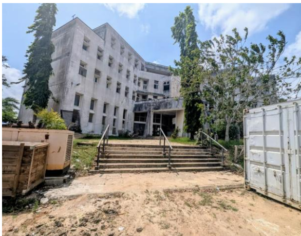
Old TAMCO building unrepaired
