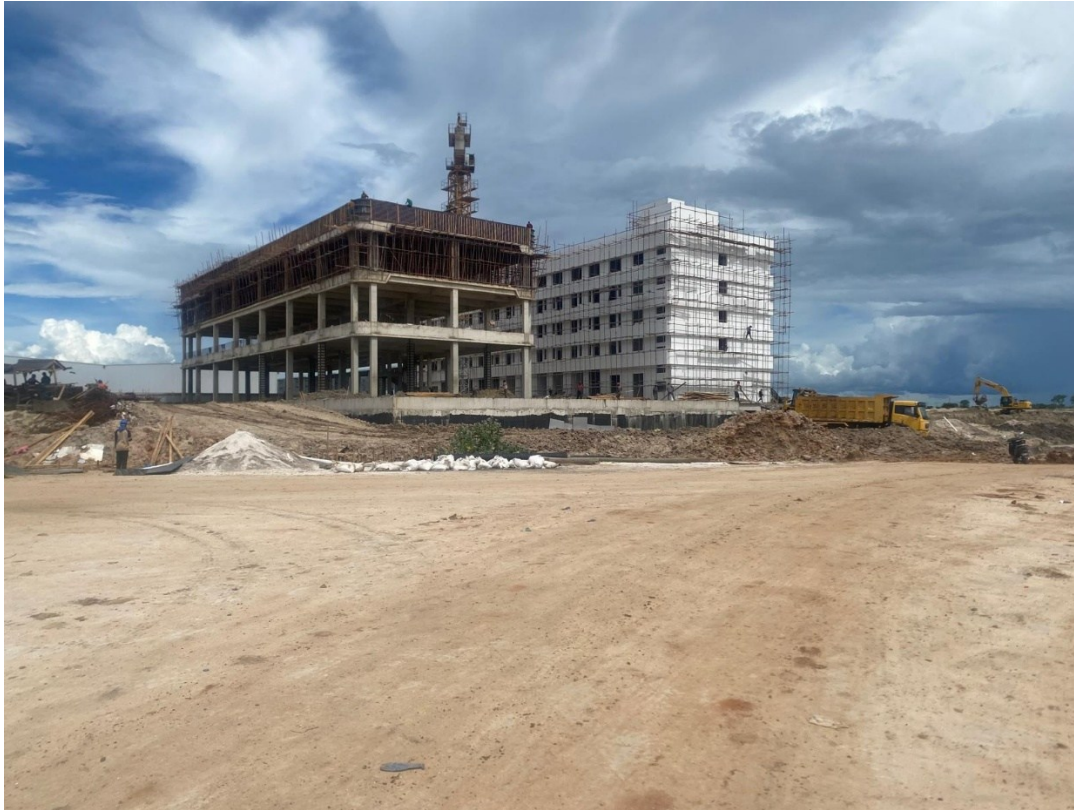
Figure 1: A picture which shows one of building which is in construction at Kwala Industrial Park
