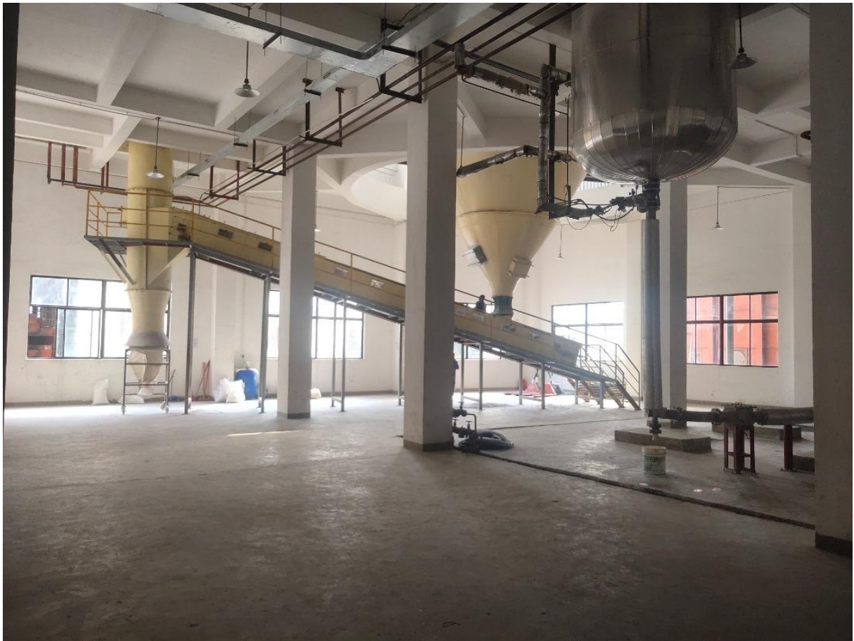
Picture No.7 washing powder manufacturing machines workshop
