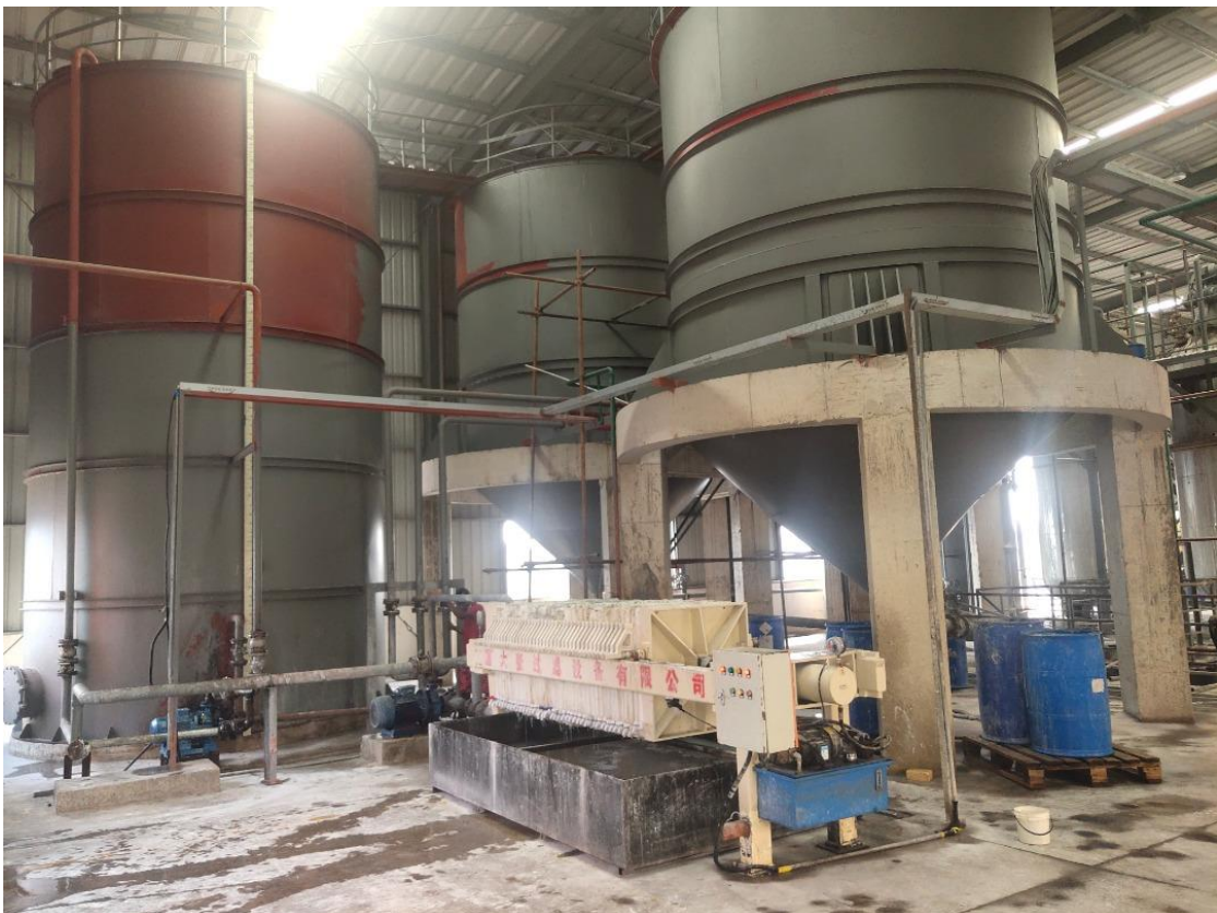
Picture No.6 Washing powder manufacturing machines workshop
