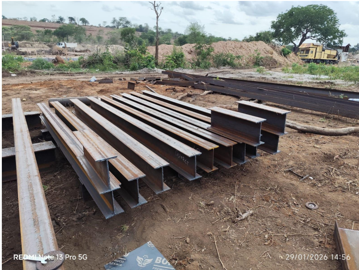
Hammer crusher structure
